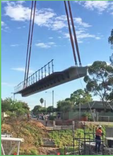
The span of the new Hallett bridge along the River Torrens Linear Park being lowered into place. The bridge was completed in April 2016. Photo courtesy of: DPTI SA
