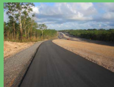
An 8.6 km long shared path was built on Tiger Brennan Drive, Darwin
